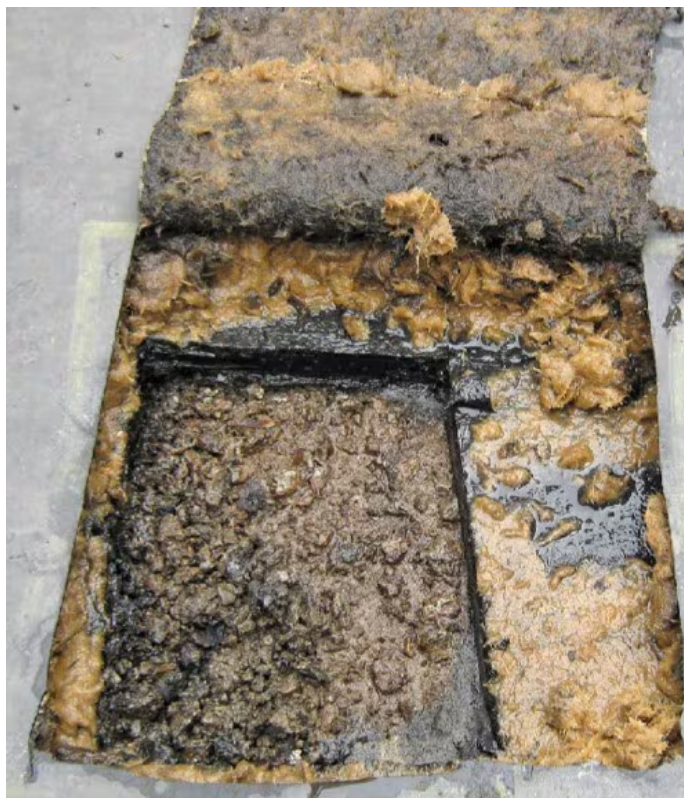
Figure 3. Moisture trapped between two Class I vapor retarders caused degradation of the insulation and roof deck (Image courtesy of SGH).
