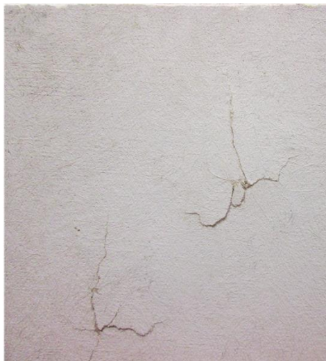
Cracked underside on a gypsum board
